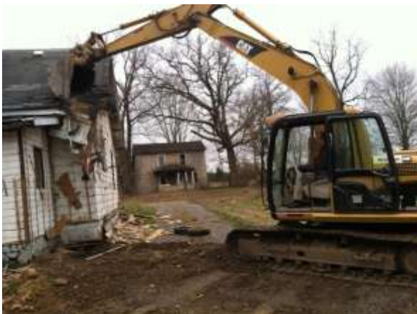
Demolition of structures on Woodville Road. Kent Maurer in the driver’s seat.
