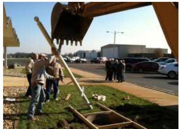
Installing the mounting pole in front of the terminal building in anticipation of the WWI replica airplane.
